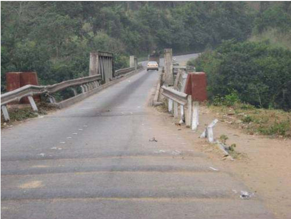
Plate 1.22: Narrow Bridge Along the Makeni Freetown Route. The Conductor Rails Need Replacing.
